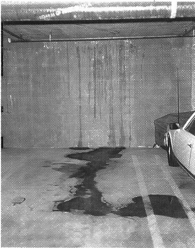
Left: One of the first signs of defects in construction is water damage. (Photo courtesy of CBI Construction, Las Vegas.)
